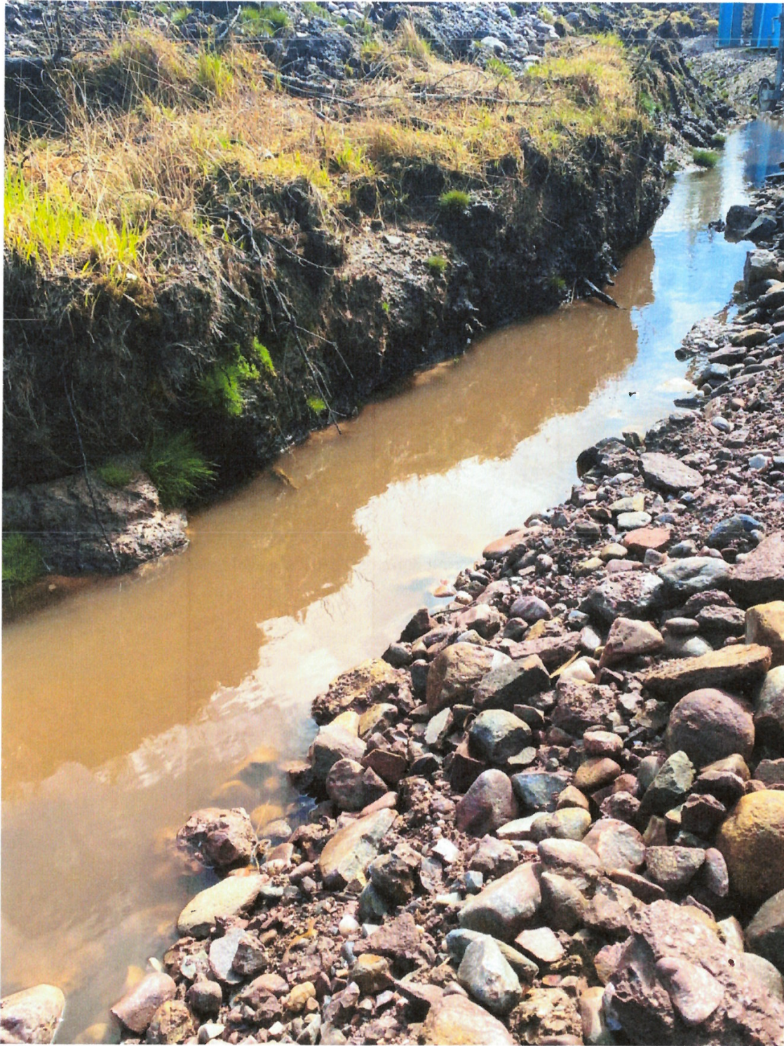
Figure 12. Muddy runoff channel along the southside of the main area of works onsite.
